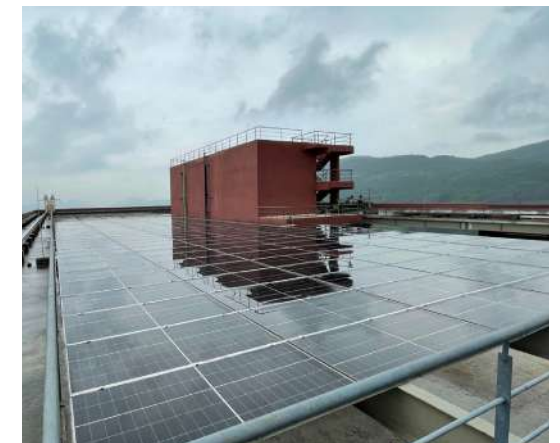
Fig. 4.17 Canopy. Source: Aelius Turbina.
